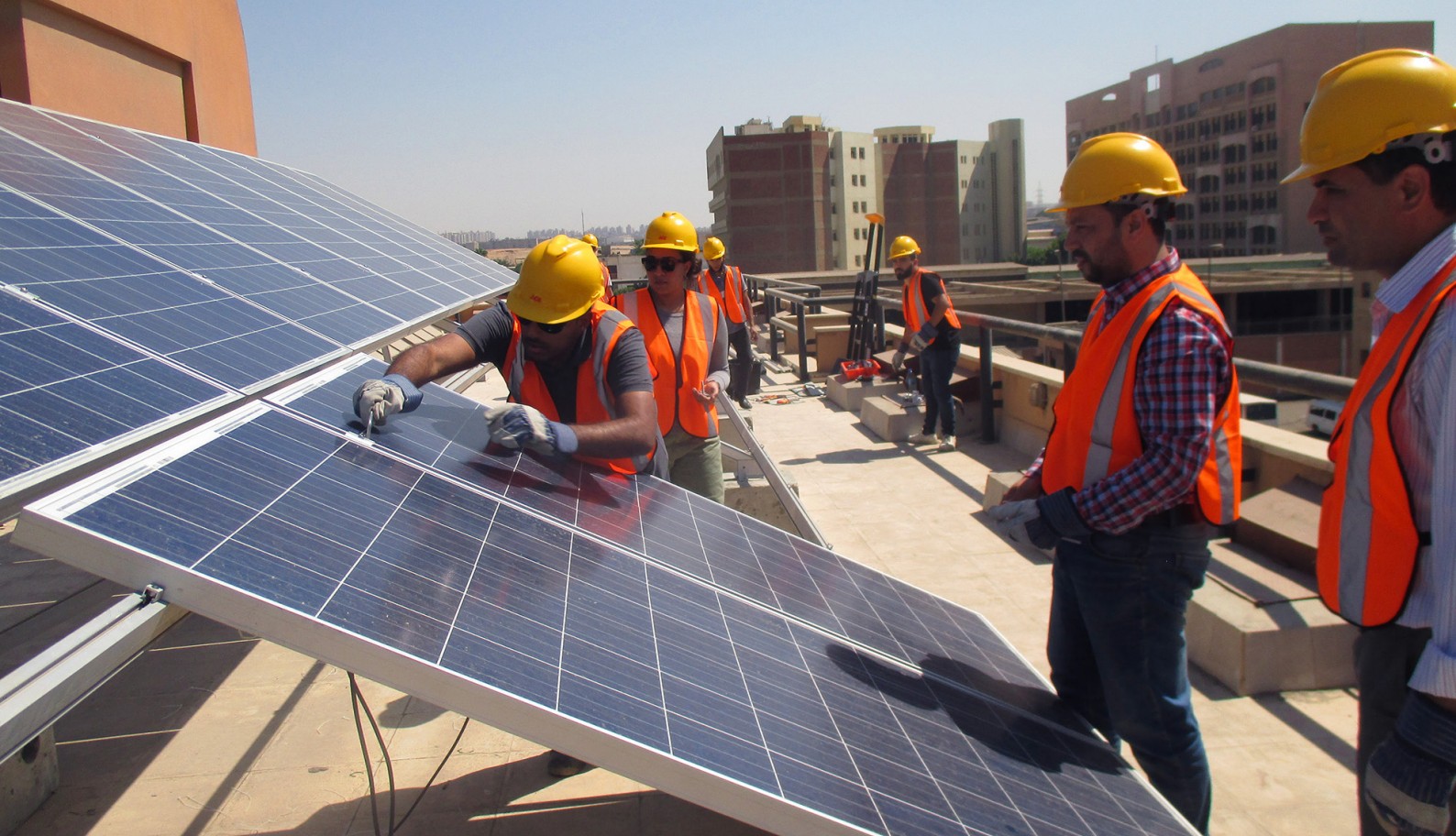
PV module installation within a training for grid-connected PV in Cairo, Egypt © RENAC
